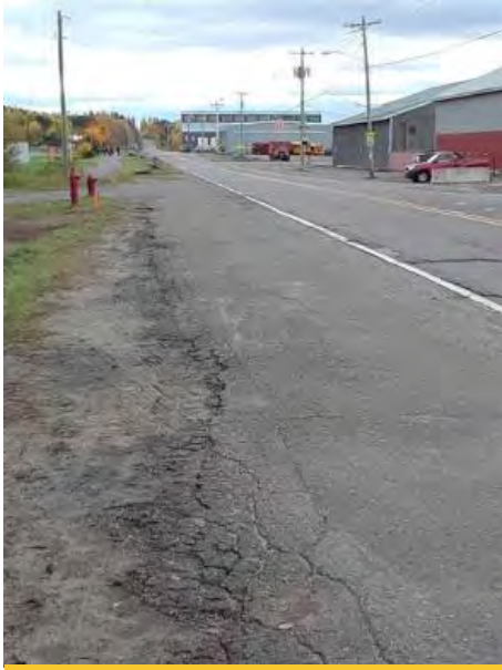
Shoulder becomes unpaved near the intersection.
